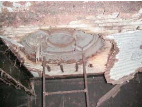
Support tin rusted & concrete deteriorating
