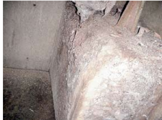
Concrete Support Deterioration
