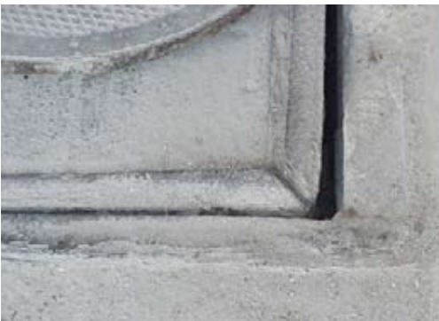
Scale deck rubbing from coping rust
